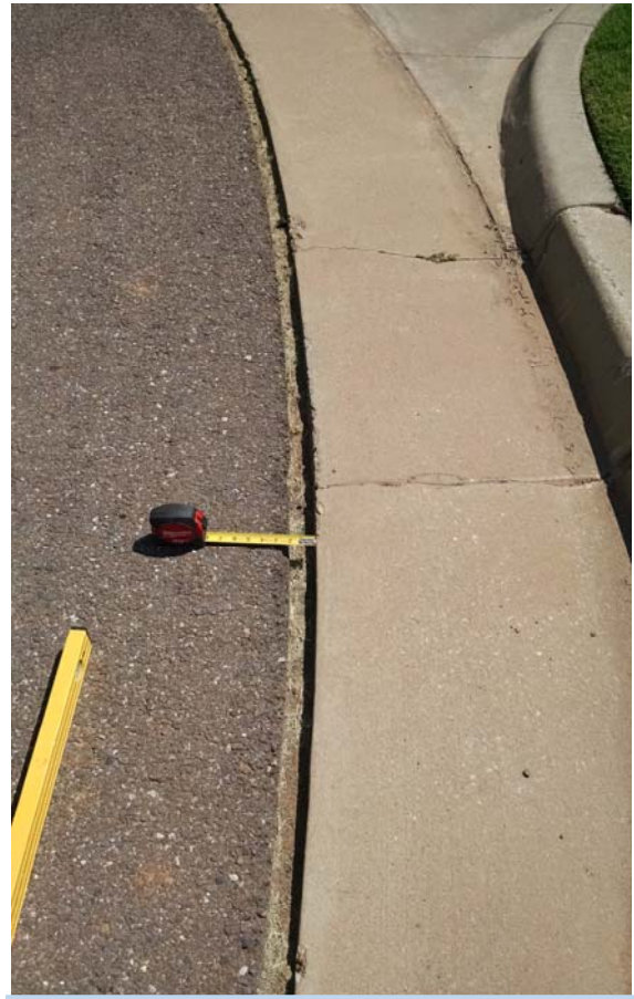
SEPARATION AT GUTTER JOINT
