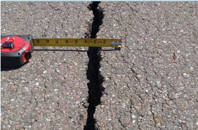
MAJOR TRANSVERSE CRACK
