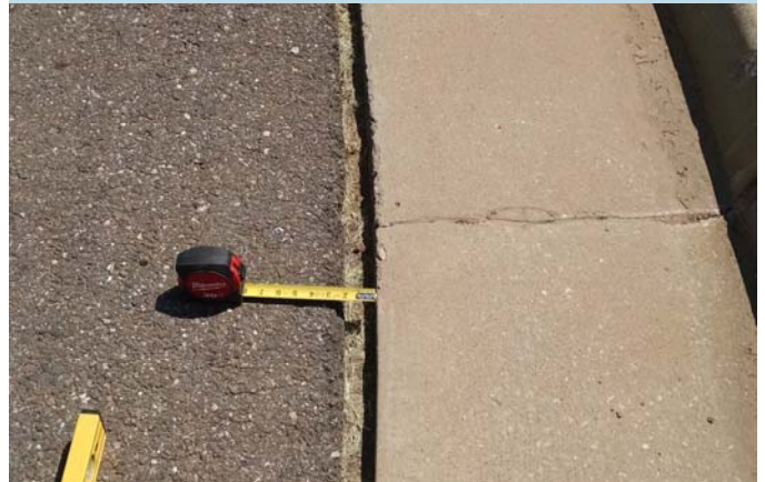
SEPARATION AT GUTTER JOINT
