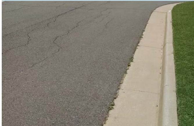
MINOR CRACKING AND RAVELING
