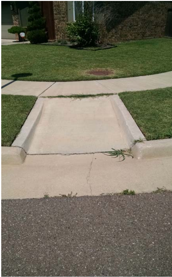
NON COMPLIANT WHEEL CHAIR RAMP
