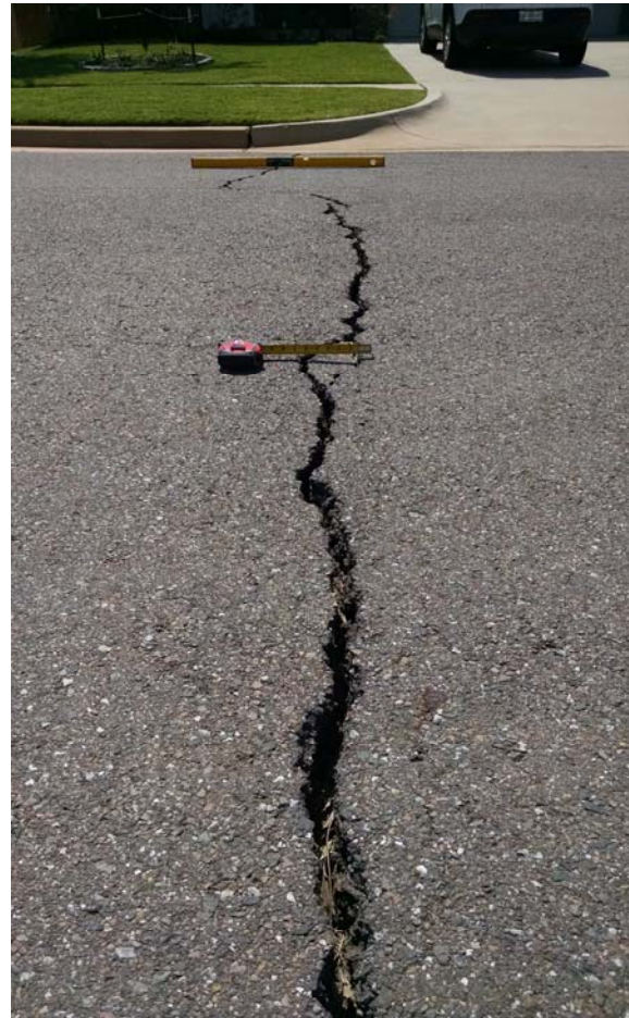
MAJOR CRACK (BLOCK JOINT REPAIR)
