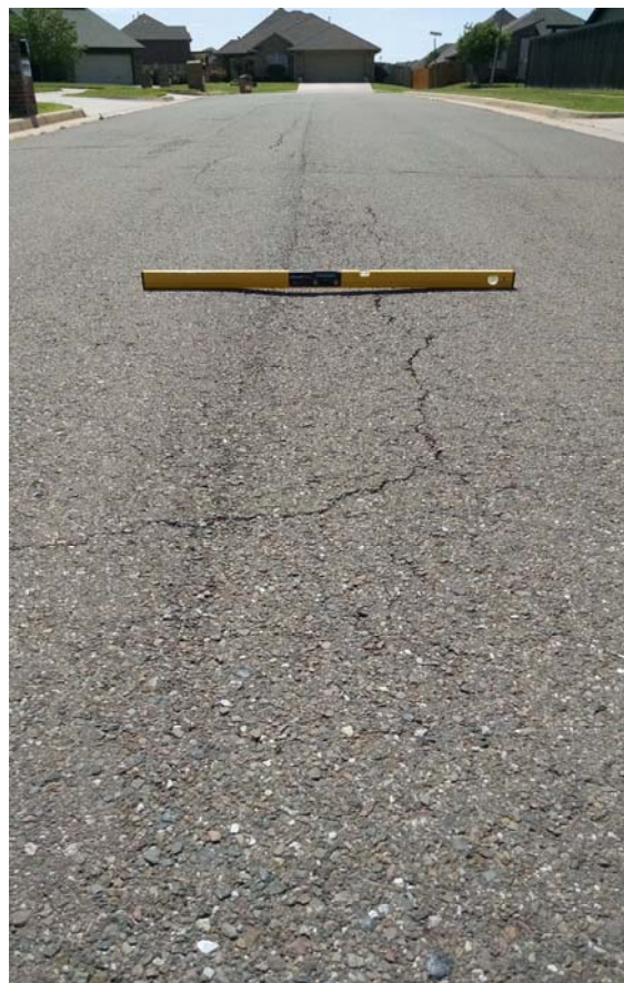
MINOR CRACKING AND PAVEMENT PROFILE
