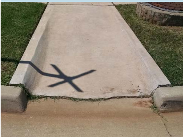
NON COMPLIANT WHEEL CHAIR RAMP
