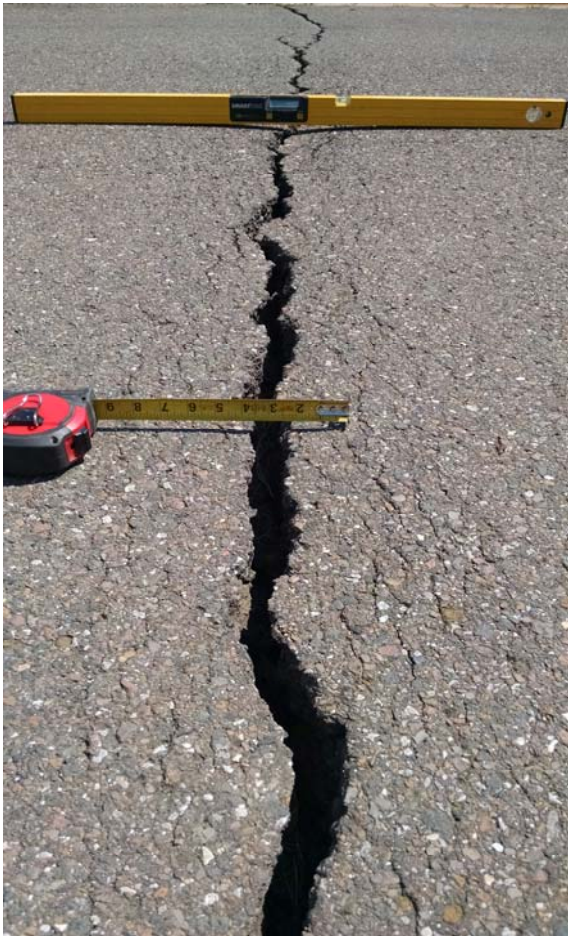
MAJOR CRACK (BLOCK JOINT REPAIR)
