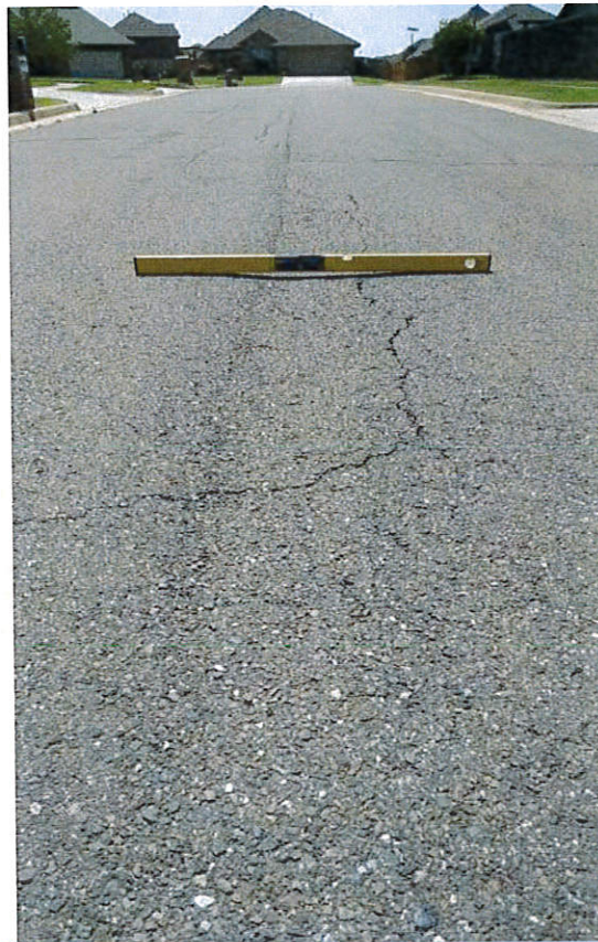
MINOR CRACKING AND PAVEMENT PROFILE
