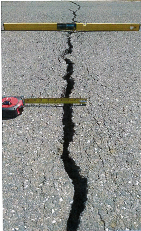
MAJOR CRACK (BLOCK JOINT REPAIR)
