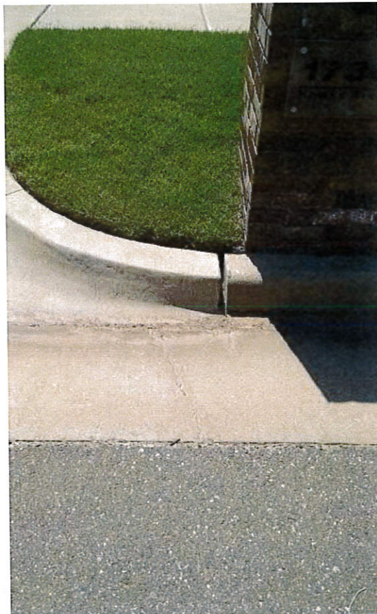
DRIVEWAY SEPARATION AND GUTTER CRACKING
