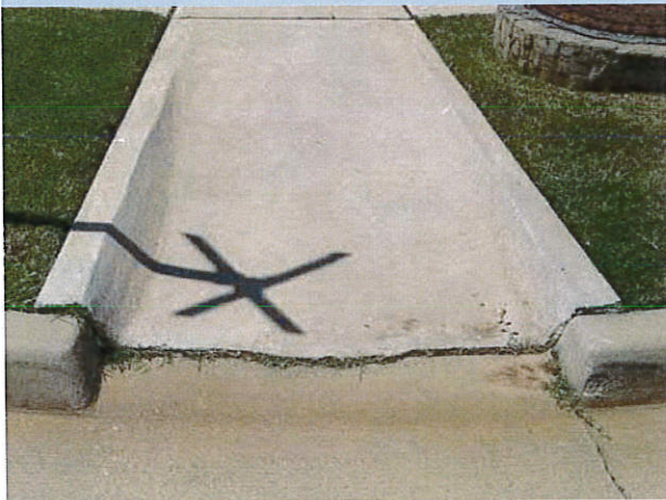
NON COMPLIANT WHEEL CHAIR RAMP
