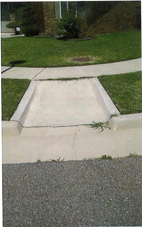
NON COMPLIANT WHEEL CHAIR RAMP
